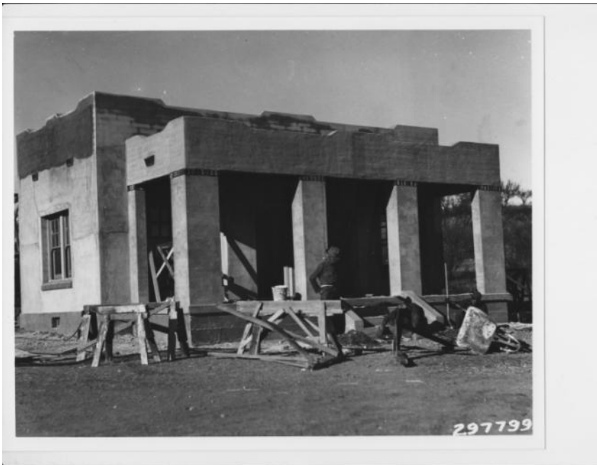
Figure 6. Coronado National Forest, Arizona. Office building under construction at Patagonia Ranger Station. Work by Flux Canyon ECW Camp F-63-A. Photo by Lee Kirby. Nov. 1934. #297799. (Courtesy William B. Gillespie)
