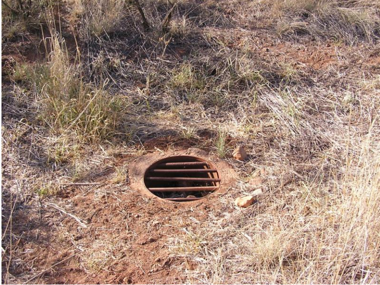
Figure 5. Drain at bottom of earthen dam, downstream side, CCC Canyon, town of Patagonia. (S.E. Hunt)
